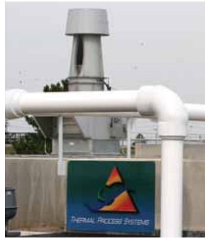
BiofiltAer with exhaust fan
