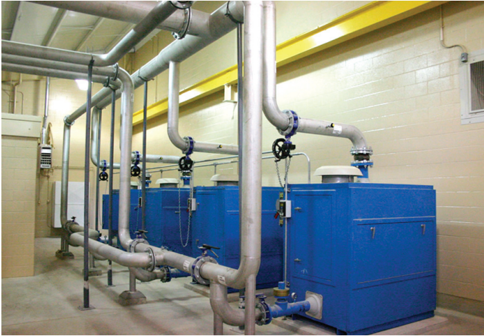
Blowers provide the oxygen required by the system as indicated by the ORP.
