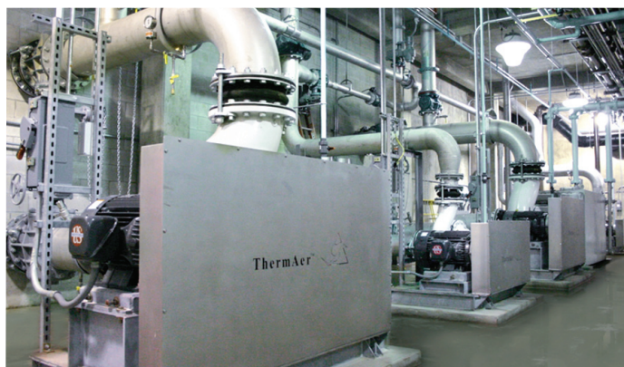
Out-of-basin pumps complete with VFDs allow for variations of mixing intensity.
