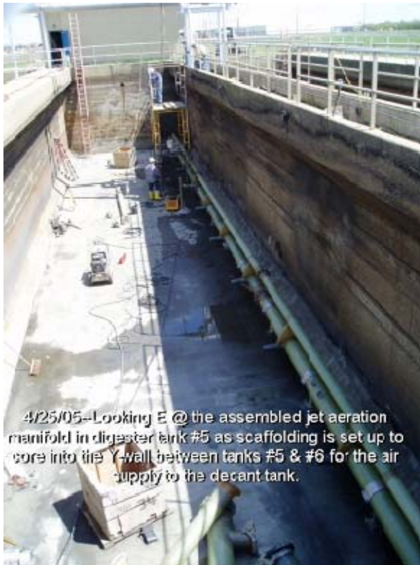
Figure 8 Liquid Aeration/Storage Tank
