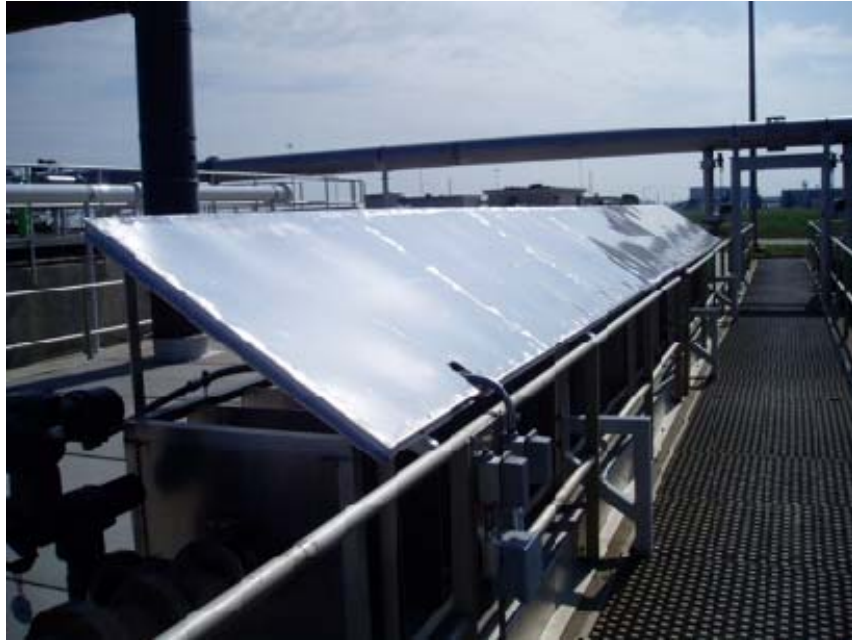
Figure 10 Passive Radiator with Sun Screen
